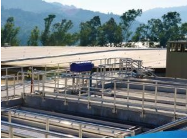
The San Jose Water Company revitalized its largest surface
